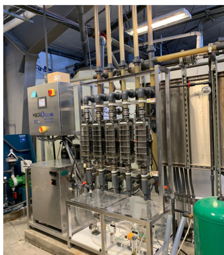
Chlorine Generation System
